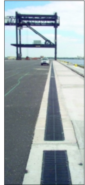
Port Trench Drain
